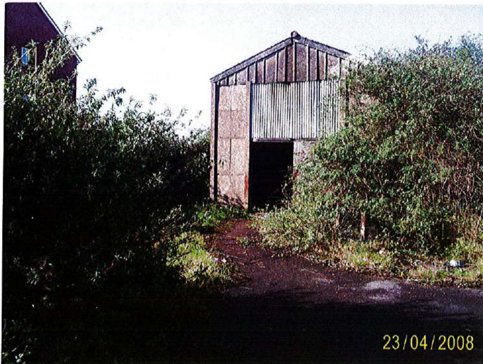
Photograph 4: Photograph showing derelict building in south-eastern section of the site. Concrete tank supports (location of TP1) visible within overgrown vegetation in right of photograph.
