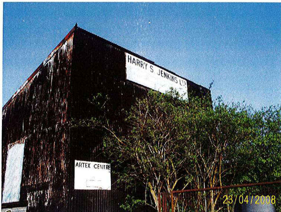
Photograph 1: Photograph of derelict building located in the north-eastern section of the site, taken from Coverack Road. Photograph shows signage indicating historic land use (Paint & Putty Works).
