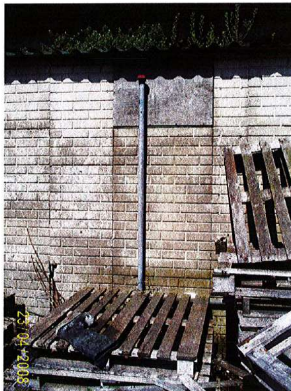
Photograph 10: Photograph showing a potential venting pipe located on building in north-western section of the site.
