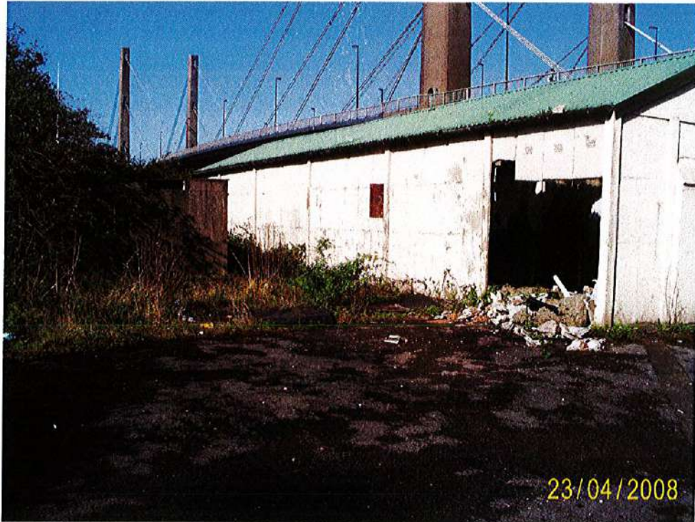
Photograph 3: Photograph showing derelict building in southern section of the site. George Street Bridge visible in background.
