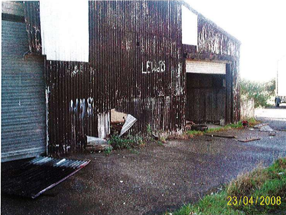
Photograph 7: Photograph showing derelict building within north-eastern section of the site.
