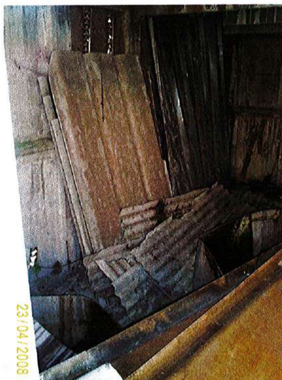
Photograph 6: Photograph showing potential ACM within derelict building in southern section of the site.
