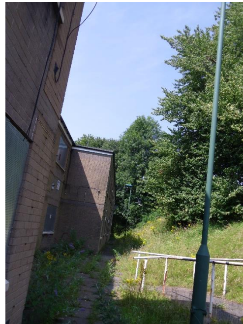
Figure 6 - Building, hardstanding, amenity grassland and scattered trees on eastern boundary of building
