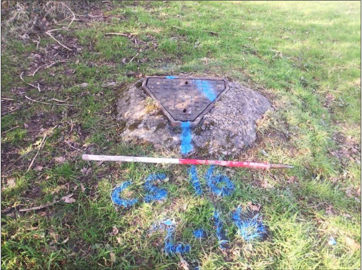
Plate 2. One of a series of raised manholes located adjacent to the Sites southeastern boundary, looking west.
