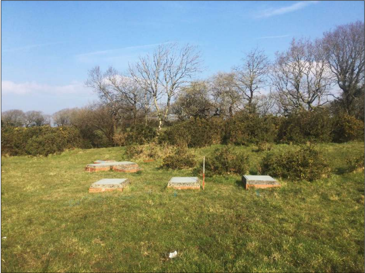
Plate 3. The northern most group of raised manholes located within the Site confines.
