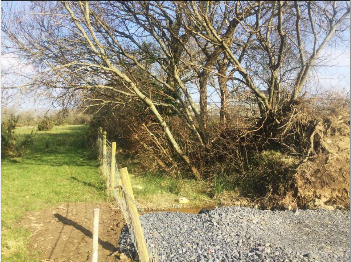
Plate 13. The southern end of the hedgebank, now terminated by modern construction road, looking north.
