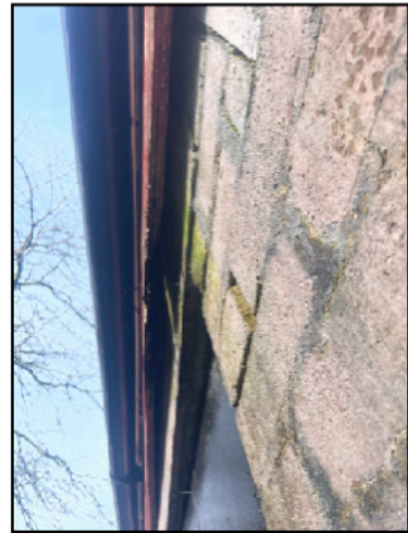
Areas of Raised Timber Fasciae on the Garage Block
