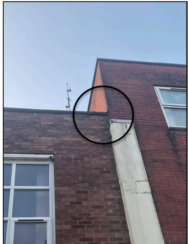
Small Area of Raised Lead Flashing to the Southern Elevation of the Extension
