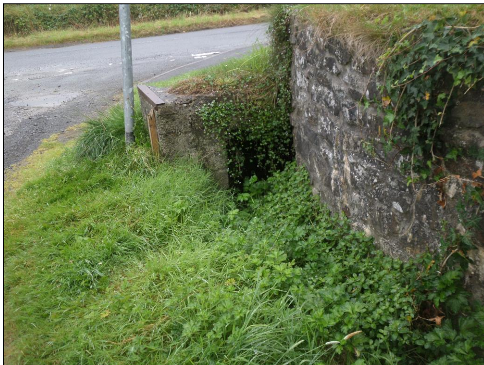
Photo 6: Running ditch flowing into culvert beneath Cwrt Melin road (view looking south).
