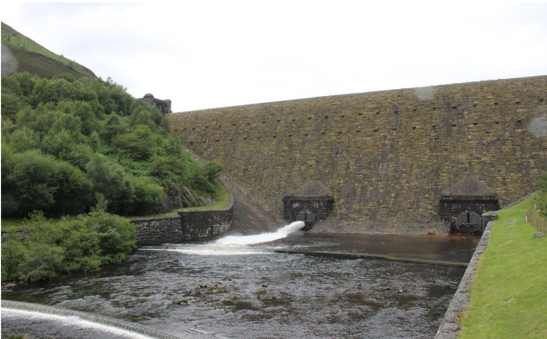
Image EDP A1.2: View of Caban Coch Dam from the bridge to the east and illustrating its appearance from the river valley bottom.
