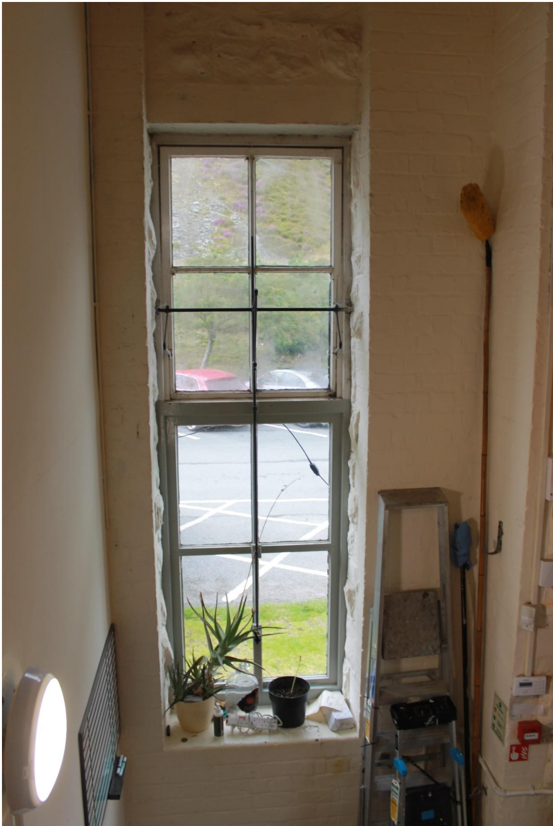
Image EDP A1.29: Internal view of one of the windows showing the preserved ironmongery of the pivot mechanism.
