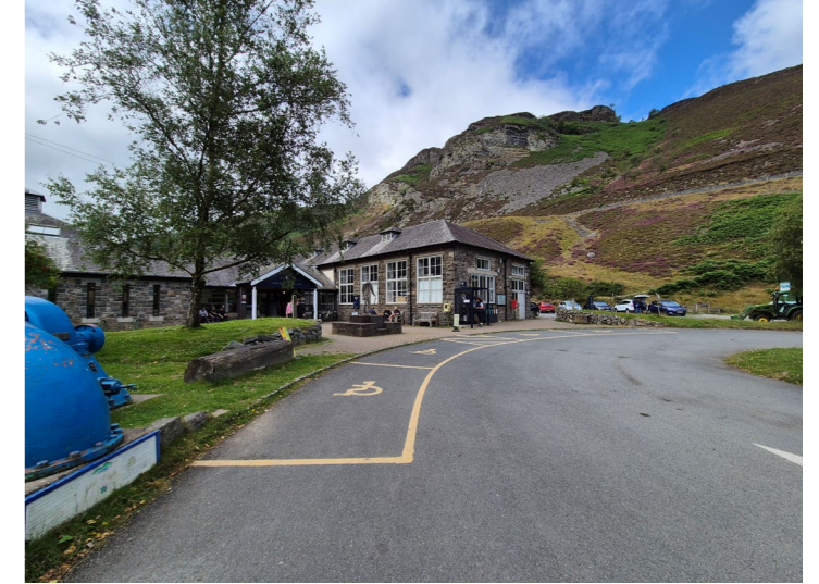
Accessible carpark obstructing welcome area and not as per standard
