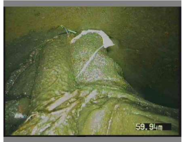
5-1-12A, 00:10:10, 59.94 m Survey abandoned, NEEDS MORE CLEANING
