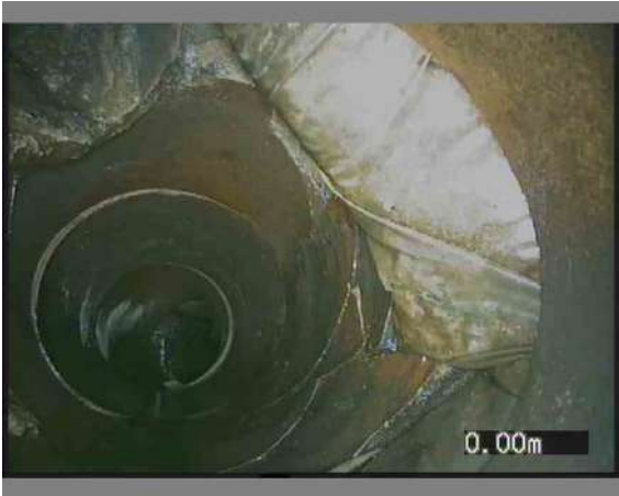
2-1-3A, 00:00:12, 0.20 m Fracture, multiple at joint, from 7 to 5 o'clock
