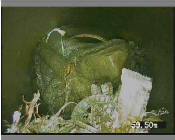
5-1-11A, 00:10:04, 59.94 m Junction at 10 o'clock, diameter: 150mm, STEEL ROD THROUGH GULLY HOLDING DEBRIS BACK
