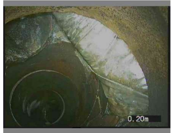
2-1-4A, 00:00:22, 0.20 m Hole in drain/ sewer, from 11 to 4 o'clock
