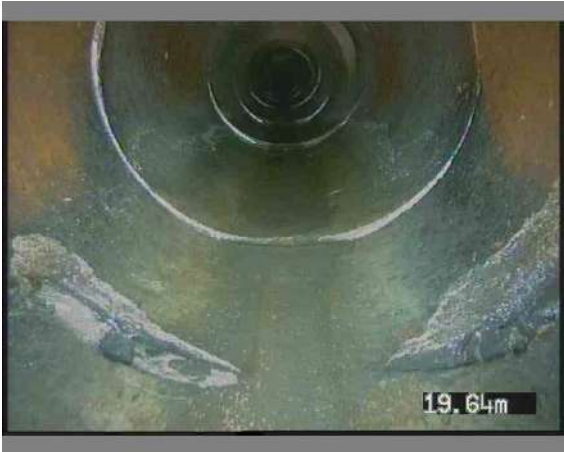
3-1-6A, 00:02:56, 19.64 m Hole in drain/sewer, from 7 to 8 o'clock
