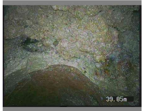
3-1-14A, 00:07:34, 39.85 m Hole in drain/sewer, from 9 to 3 o'clock
