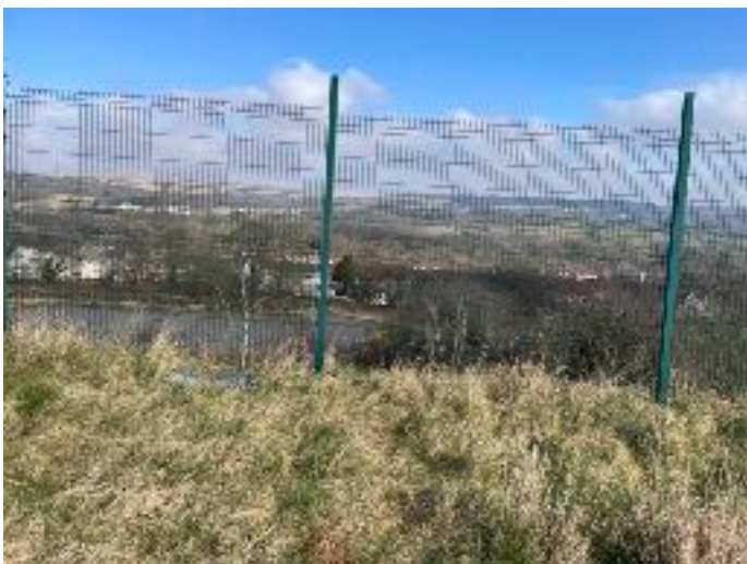
11. Large gap cut in northern boundary fence.
