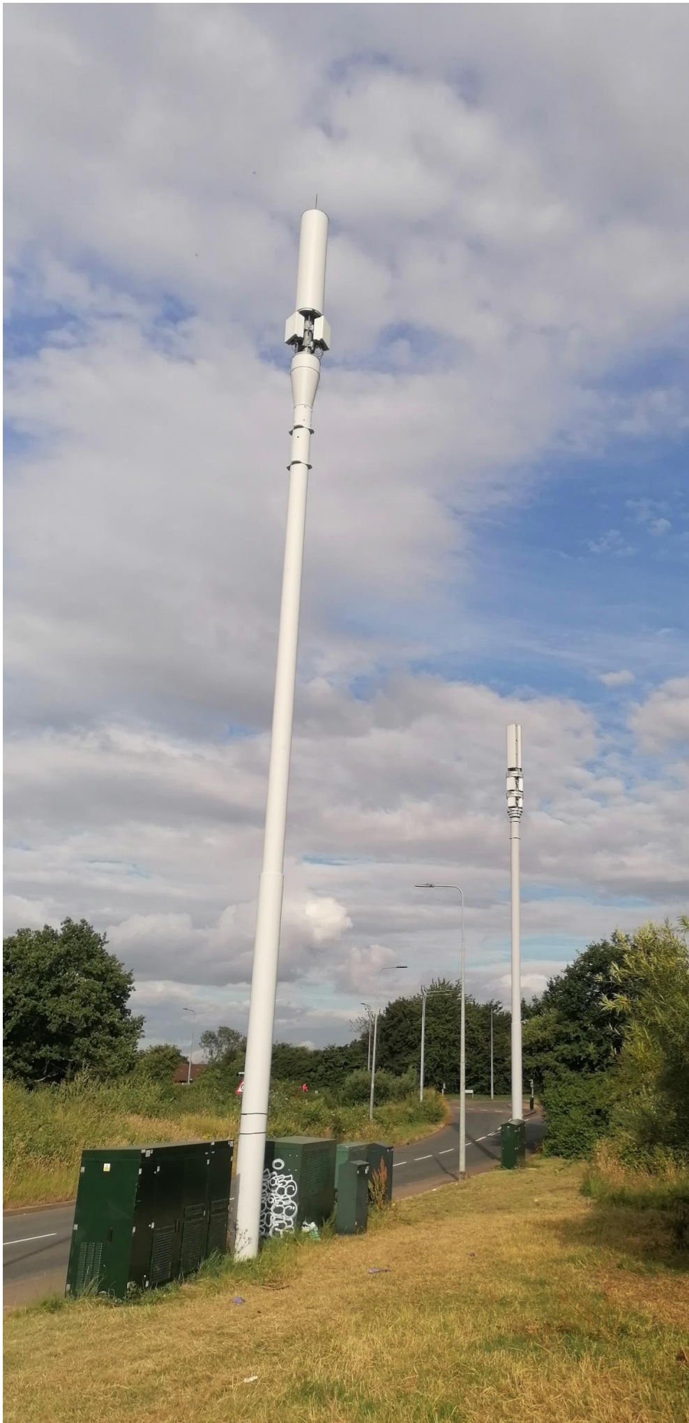
Viewpoint 3 Telecommunications masts on north-eastern boundary
