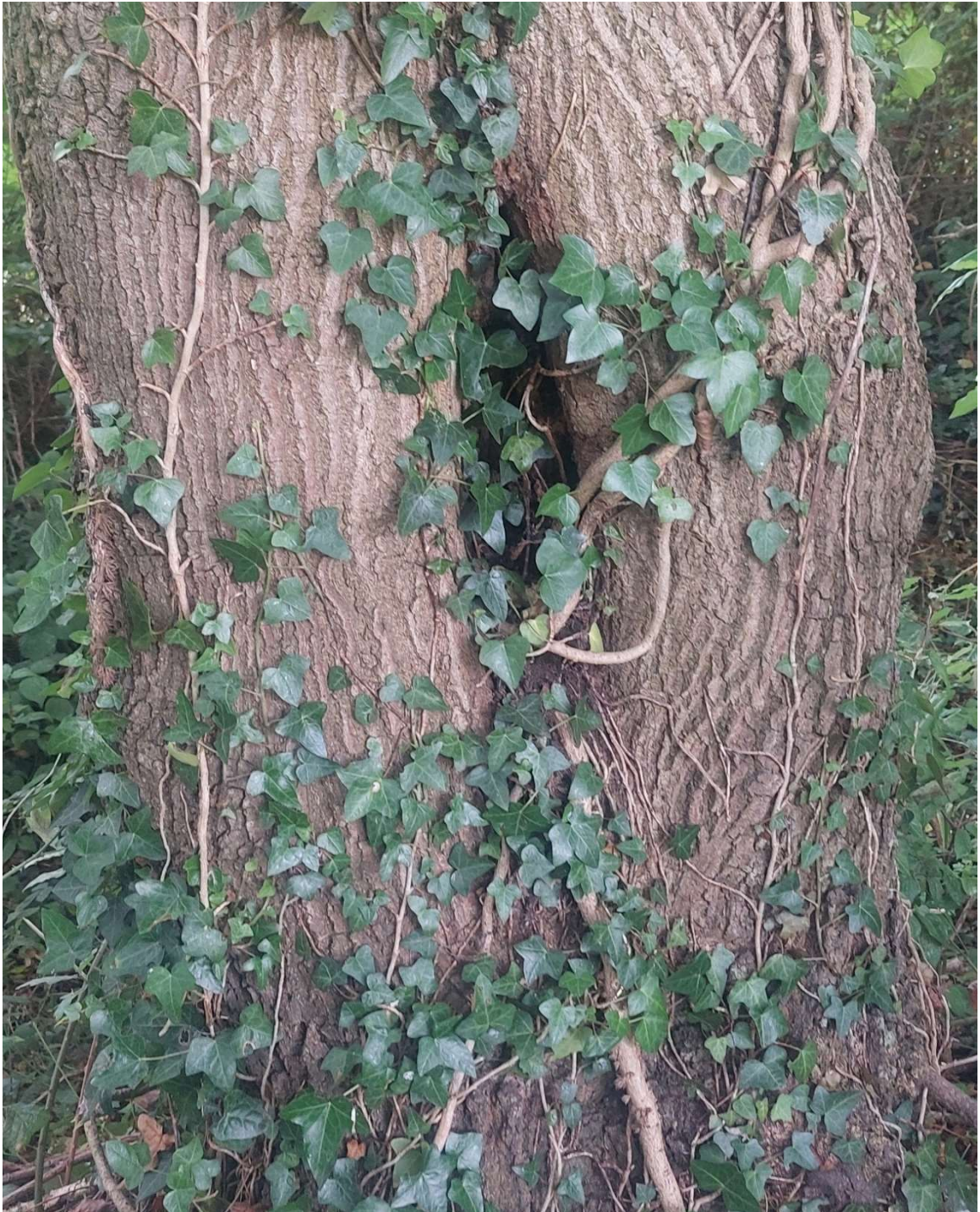
Photograph 7: T53- decay cavity and stem swelling observed at 1m above ground level.
