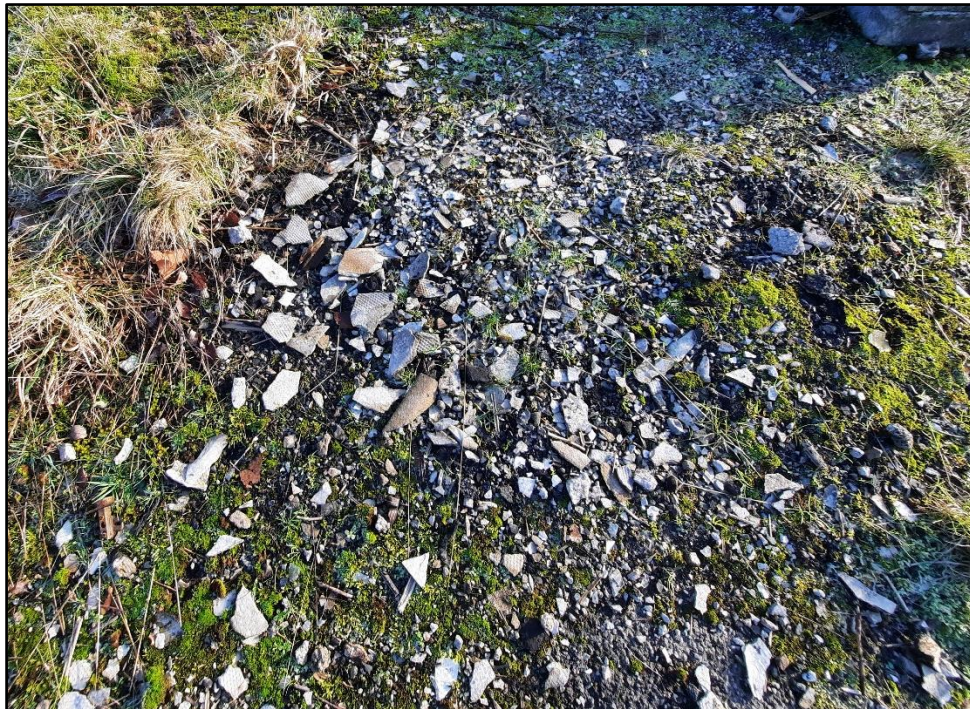
Plate 8: Fragments of Asbestos Cement Sheet on Surface, to east of Stockpile
